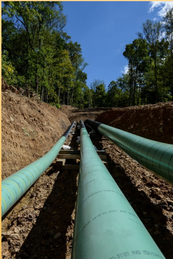
Three pipe solution at Carbide
