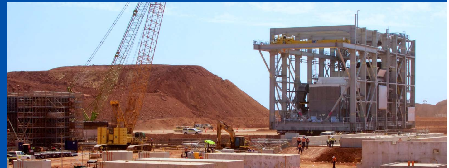
First Gas Turbine Generator
