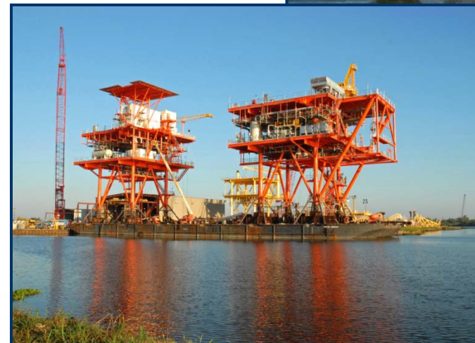
Mobilization of Production Platform for DJ #1 and Central Processing Facility for Field
