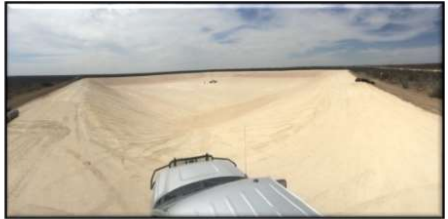
Reagan North Corridor 800,000 Bbl of Water Pit
