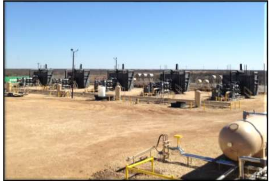
Reagan North Centralized Compressor Facility
