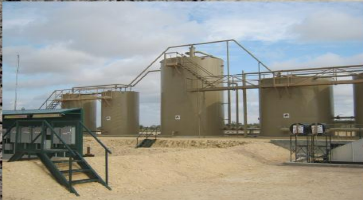
Produced water piped from horizontal wells to central disposal facility
