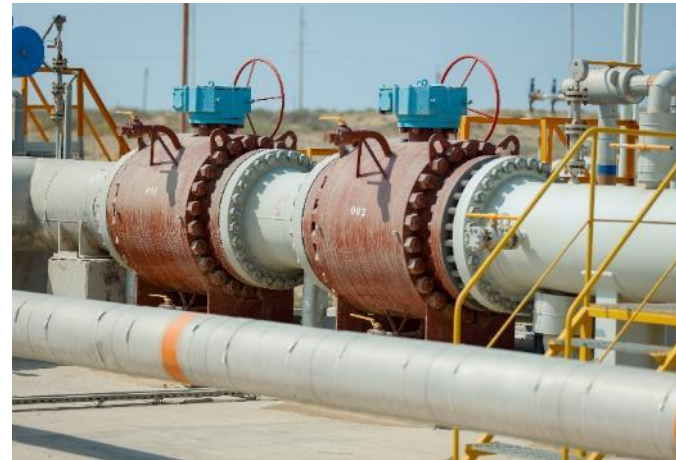
Central Processing Facility.
