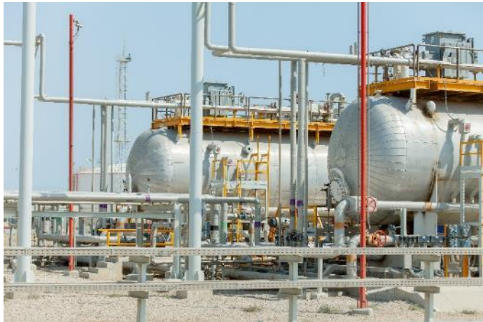
Central Processing Facility.
