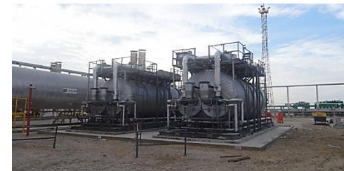
Water bath heater.
