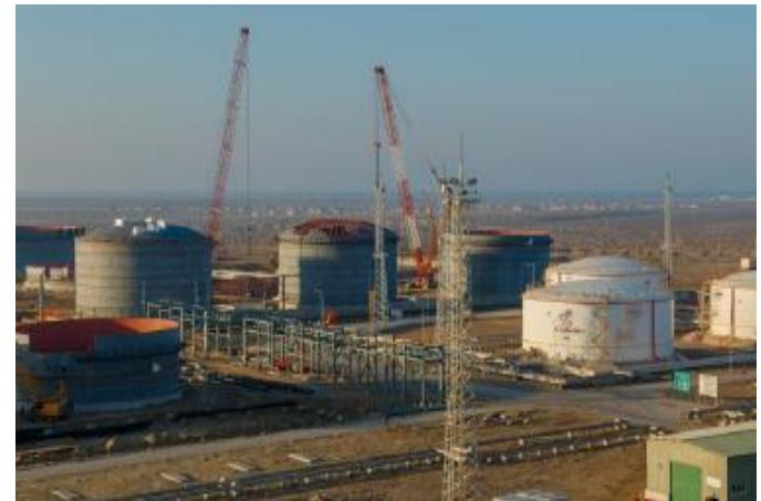
Crude oil storage tanks.
